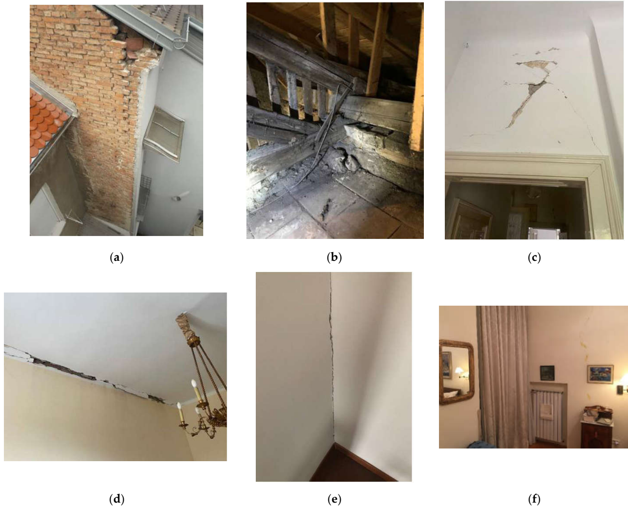
Figure 7. (a) Partial collapse of a gable wall; (b) oration of purlin's; (c) damage in the spandrels; (d) cracks at the contact of the ceiling; (e) vertical crack at the contact of two walls; (f) vertical crack along the wall [32]. Reproduced with permission from Projekt na kvadrat d.o.o., 2022.
