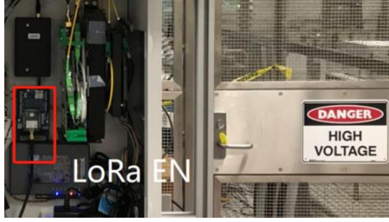
Figure 7. LoRa end node receives optical sensor data
