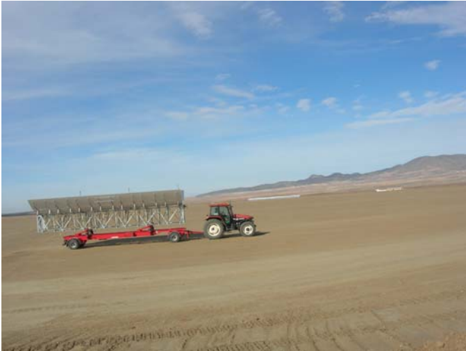
Transport of the first assembled solar collector elements on the field in Spain
