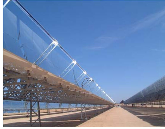
Collector in operation
