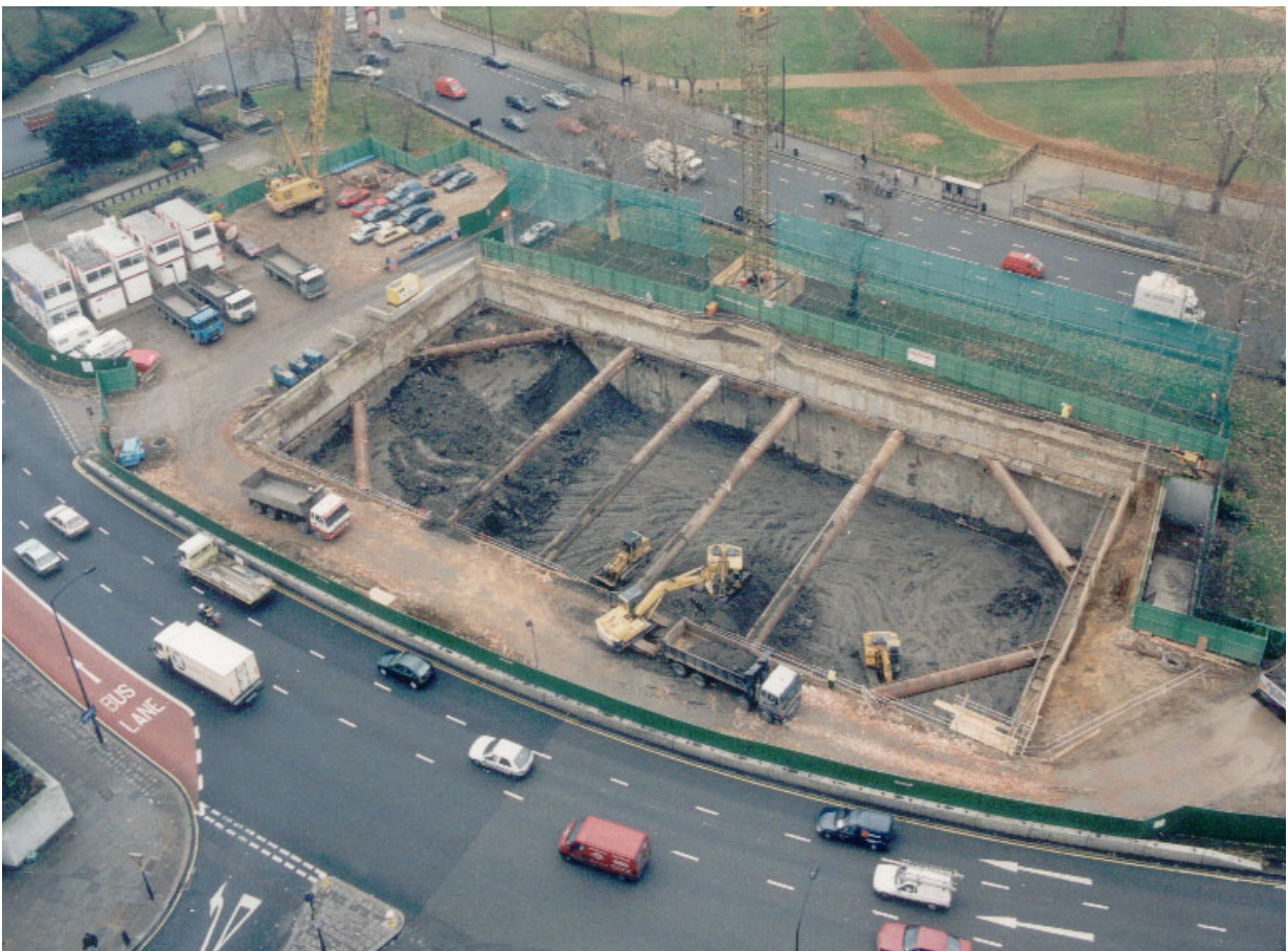
PLATE 3.6 Temporary props spanning full width of excavation for the Mayfair car park, London
