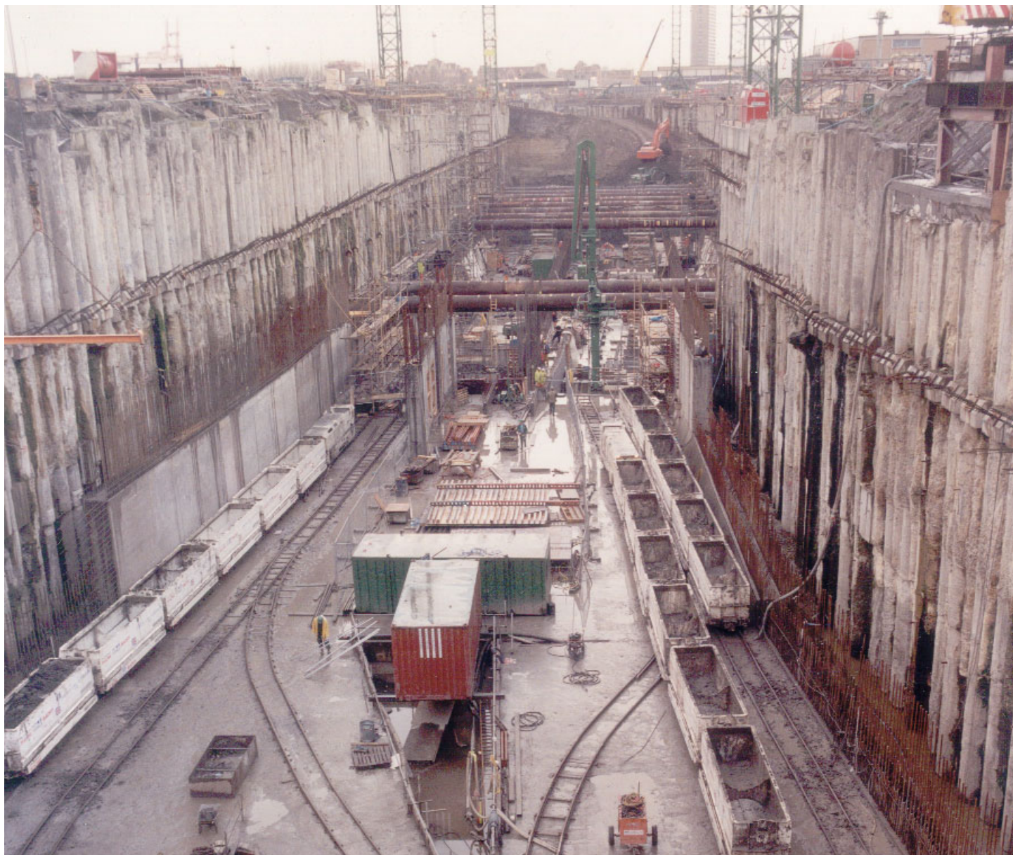
PLATEC.3 Hard/soft secant pile wall as temporary works at North Greenwich Station, London (courtesy of Bachy Soletanche Limited)
