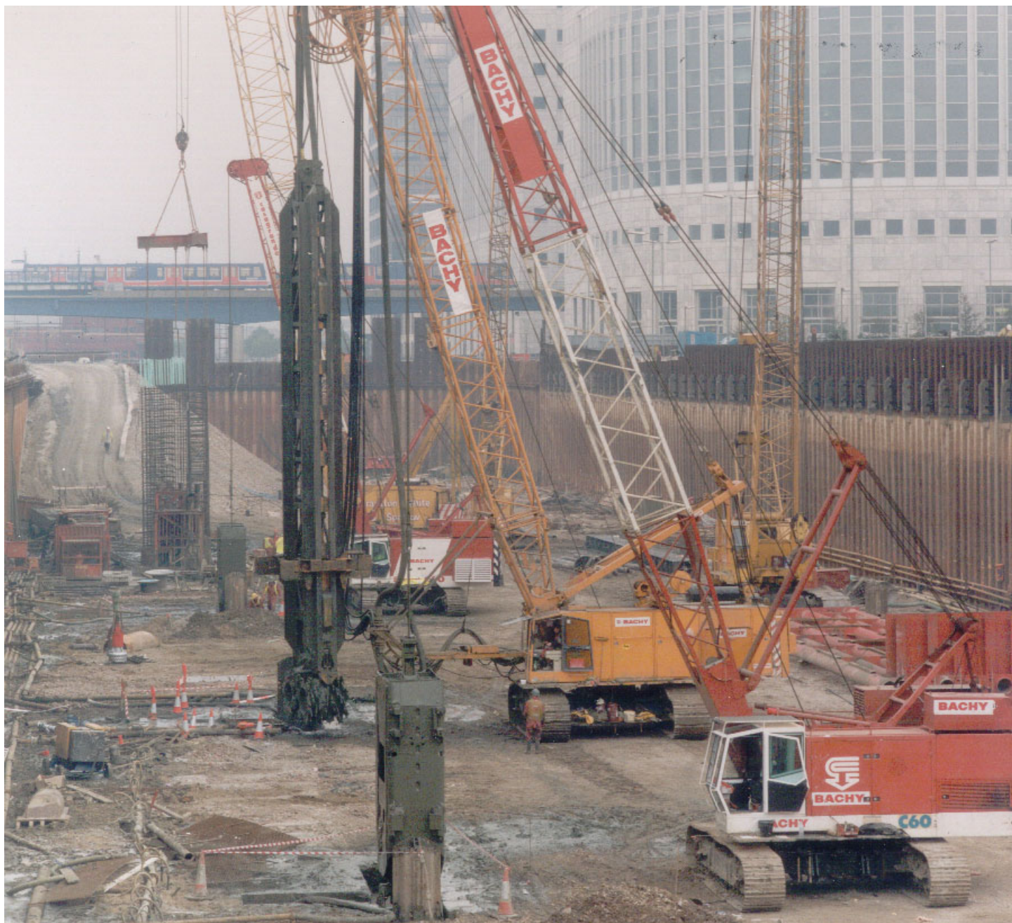
PLATE C.5 Diaphragm wall construction at Canary Wharf Station, London (courtesy of Bachy Soletanche Limited)
