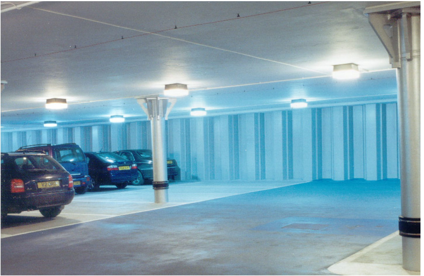
PLATE 3.1 Temporary and permanent works: Bristol underground car park. An example of the use of a sheet pile wall as the permanent wall, exposed and painted.
