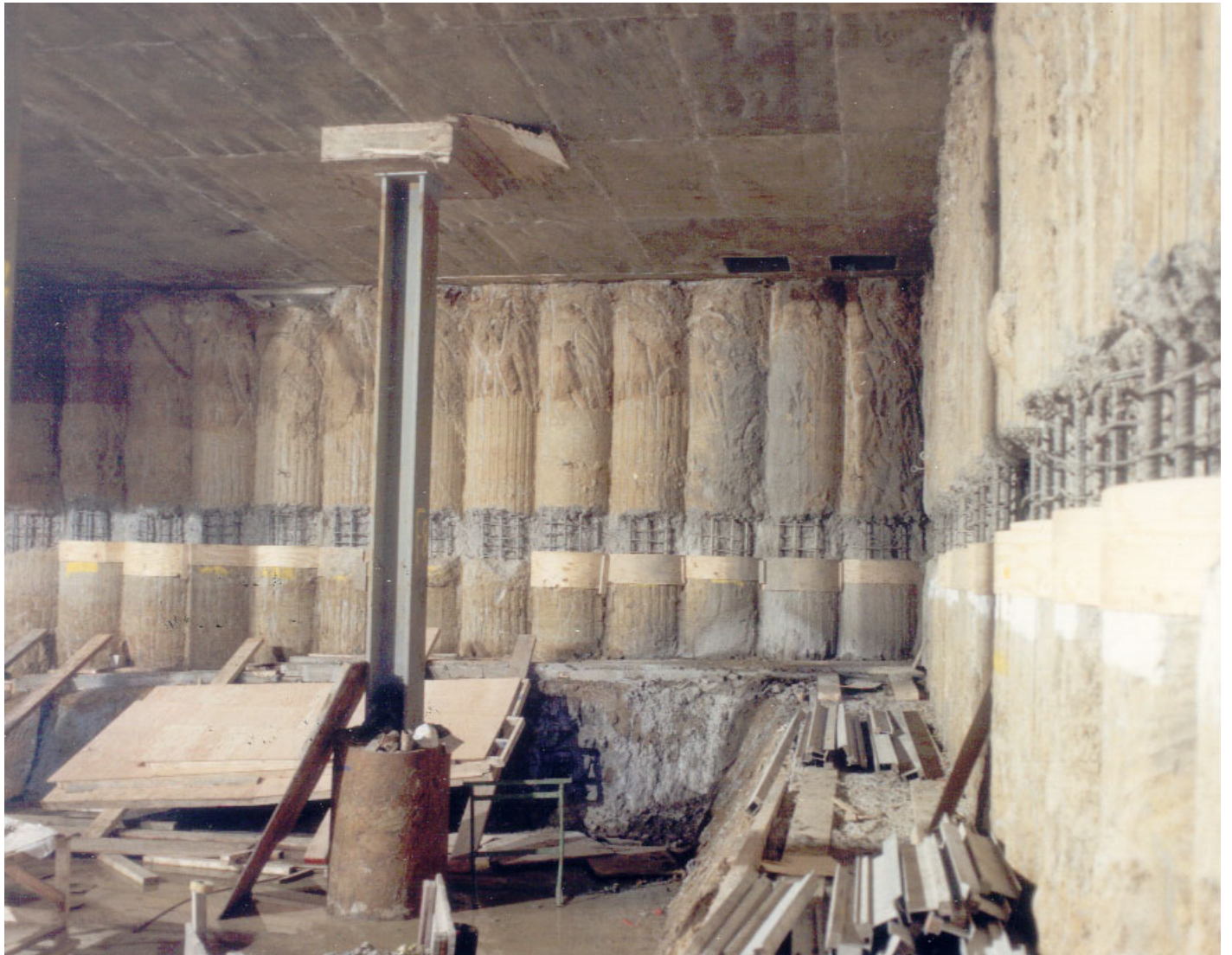
PLATEC.4 Hard/soft secant pile wall and an example of top down construction (courtesy of Bachy Soletanche Limited)
