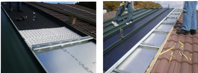
Figure 2. Installation of the PCM heat sink with reflective fiberglass insulation followed by metal roofing panels containing pre-installed PV laminates.
