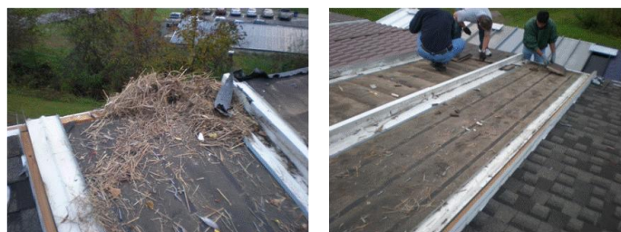
Figure 1. Cleaning of the old shingle roof and removal of old roofing materials.
