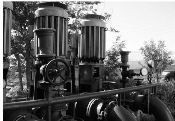
Figure 2 Details on the status of the monitoring installation
