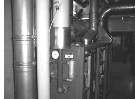
Figure 2: Microturbine installation at an office building in Munich, Germany
