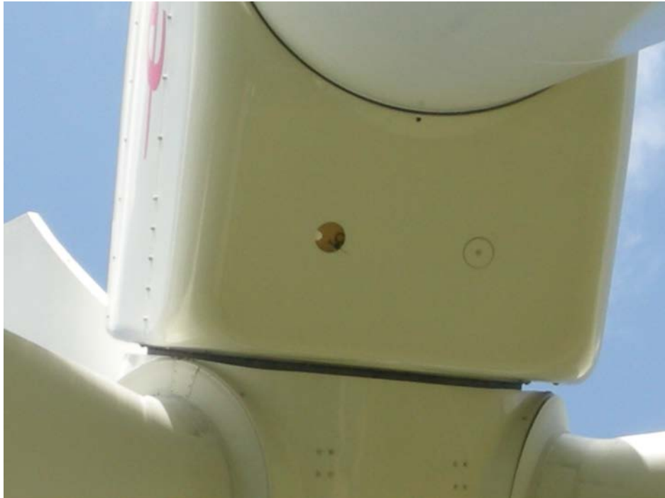
Figure 4.2 Hole in the nacelle floor between the rotor and the tower where the equipment was installed.
