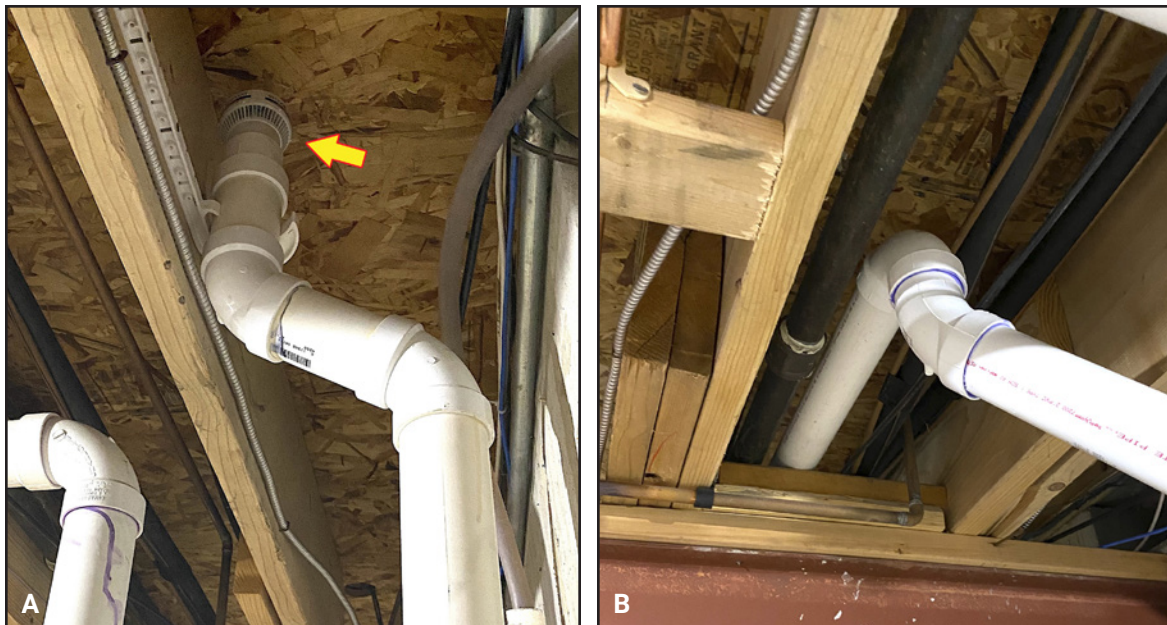
Fig. 3 Similar to leaky automobile exhaust system under floorboards, air from high-volume evacuation system may have been inappropriately exiting into utility room or basement instead of being directed outside. A. “Diffuser” exhaust for vacuum unit (arrow) was unfortunately positioned right below floor of clinic. B. Solution routes exhaust outside office.
