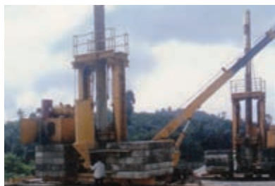
East Coast Expressway, Kerteh, Terengganu Close to 100000m of Stone Column was constructed
