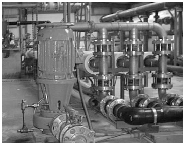
Figure 8: Work Exchanger, Handsome Bay, B.V.I.
