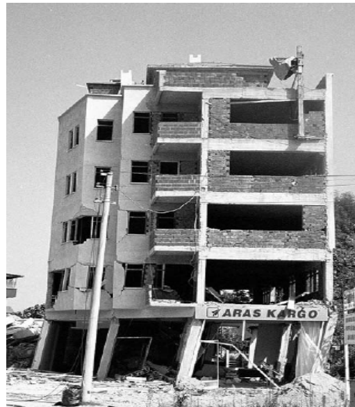
Fig.1.b Soft story failure, Bhuj 2001 [7].
