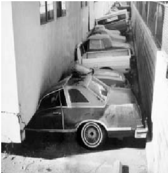
Fig.1.a Soft story collapse, Los Angeles, 1994 [5].
