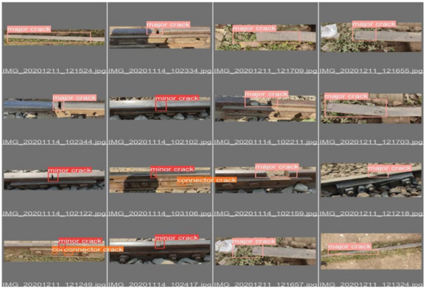
Fig. 12 Images from the test dataset demonstrating detection results of the three classes major crack, minor crack, and connector crack
