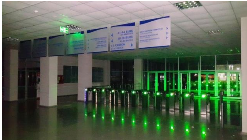
Figure 6. Main exit door emergency lighting and routing system
