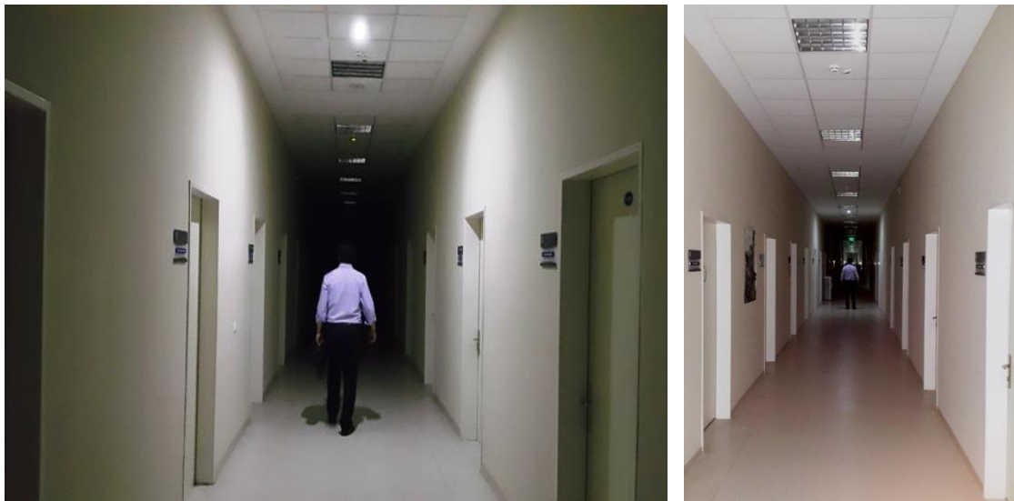
Figure 4 In the Faculty of escape routes light level and emergency lighting elements with sensors.
