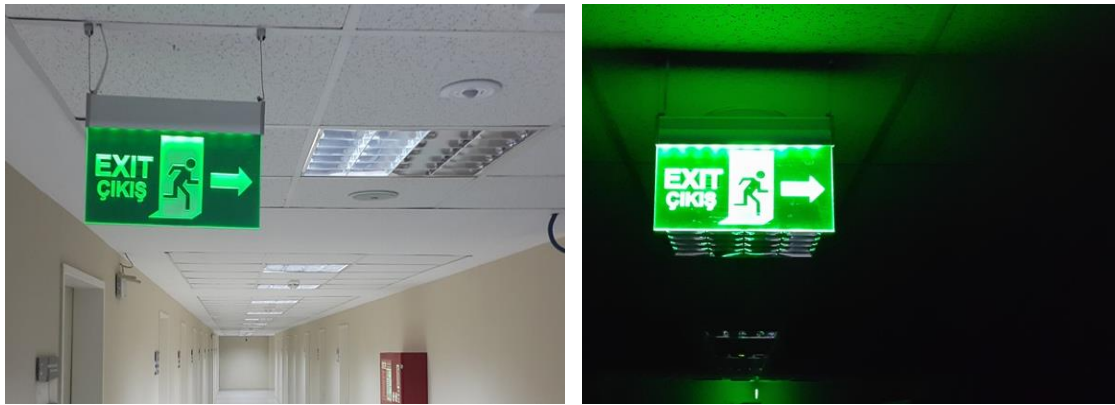
Figure 3. Emergency exit signs, bright and dark appearance.
