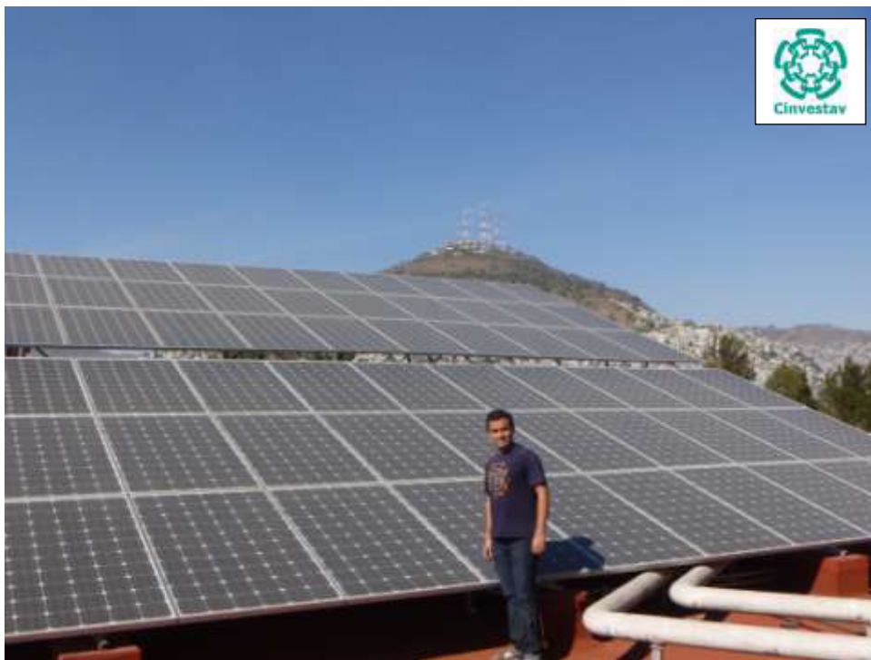
Fig. 1. Part of 60 kWp system PV module array. Each PV module consists of 250 Wp power unit, and total of 240 modules connected to 5 inverters. (Chiquihuite's mountain can be seen at the North direction at the back; 2730 meters high over sea-level)
