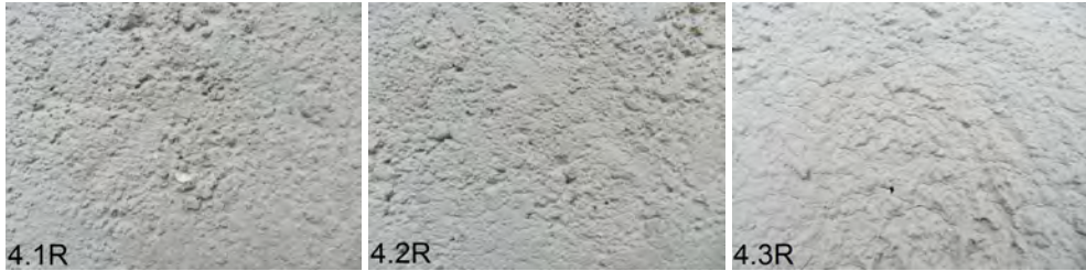
Figure 9.38: Surface cracks in finishing surface of elements 4.1, 4.2 and 4.3 (from left to right, image scale circa 16 x 12 cm)
