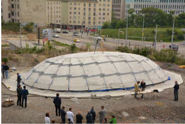
Figure 2.5: Thin concrete elements lifted by inflation of a pneumatic formwork (TU Wien, 2014)
