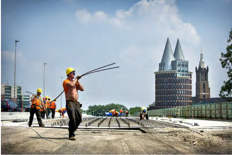
Figure 8.9: The natural deflection of steel bars - clearly visible here - is a function of diameter, self weight and support positions (Maasbrug Roermond, image Peter Wijnands Photography)
