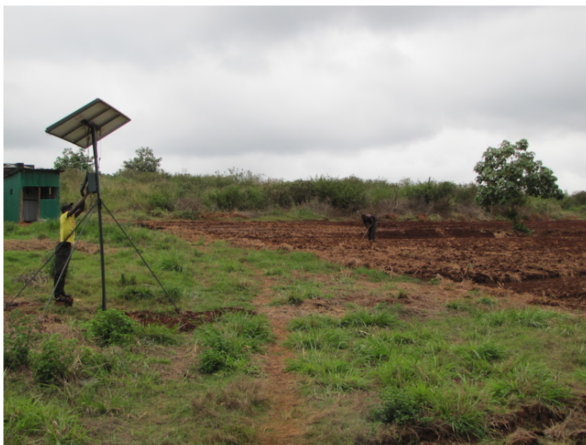
Fig. 9: Thika solar water pumping system used for drip irrigation.
