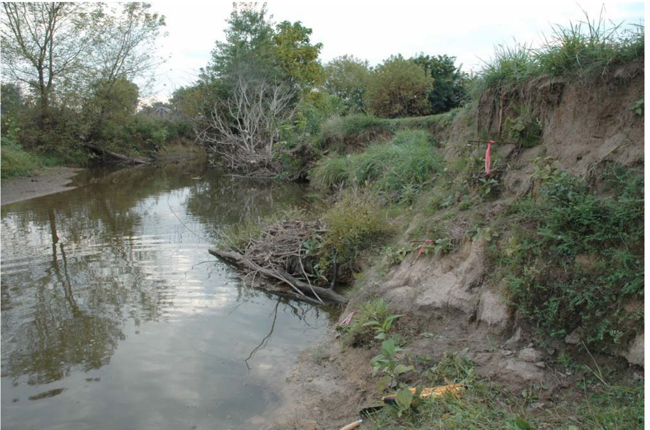
Figure 33. Right bank, Conoy Creek, showing three bank pins installed by LandStudies, Inc., just south of Elizabethtown, in February, 2006. A breached dam is located downstream ~600 ft upstream of a breached mill dam. Note bank pins (rebar) near top, middle, and bottom of bank, indicated by orange flagging tape. All pins were flush with the bank edge when installed, and by the time of this photo (Oct 10, 2006), the pins were exposed up to 2 ft. This is also the site of cross section 2 (shown as the second section line from the right on Figure 31a, at ~mile mark 5 on Figure 31b). Our GPS surveying of the bank edge in the vicinity in December 2006 indicates up to 40 ft of lateral erosion between 2001 and 2006. Our analysis indicates channel widening along this reach of Conoy Creek. This section of Conoy Creek is funded for stream restoration in 2007-2008 by LandStudies, Inc.
