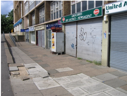
Figure 1: An example of cracked pavement
