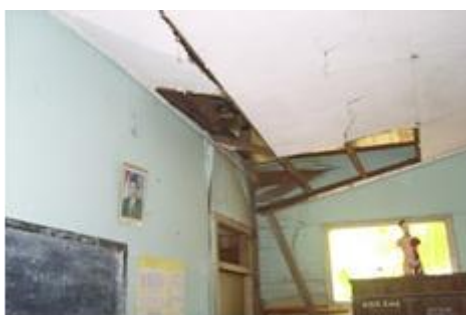
Figure 3. Damaged building where learning
