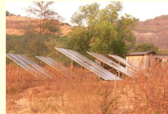
5 kWp Village power, Maharashtra
