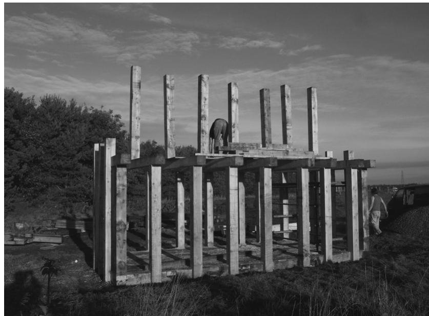
ILLUS. 43 The timber framework of uprights and lintels in place, with uprights to support the ridge pole and rafters placed in the centre of each lintel
