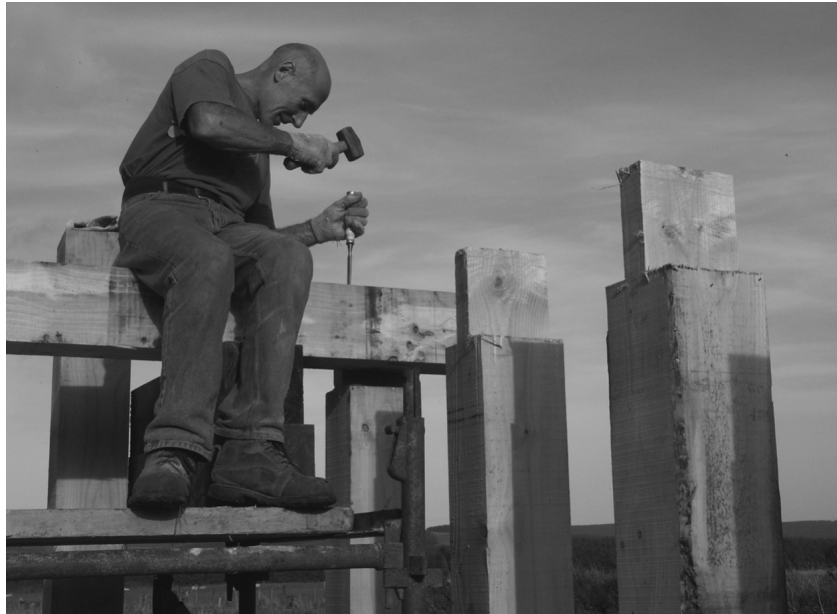
ILLUS. 42 Carpenter Peter Stapley creating a mortise-and-tenon joint to connect the timber uprights with the lintels
