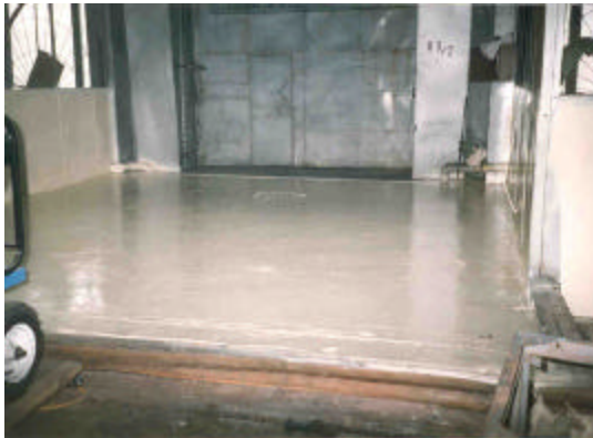
Figure 3. Concrete loading dock floor in the high bay after spray coating with Polibrid 705.
