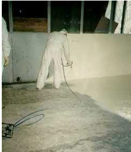
Figure 2. Russian technical expert spraying the concrete floor of the loading dock in the high-bay area.
