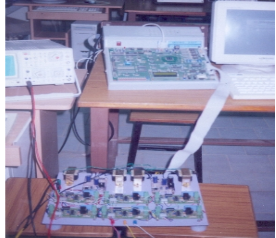
Figure 3. Hardware prototype module of extra HV dc-dc boost converter with DSP TMS320F2812 processor in closed loop operation.
