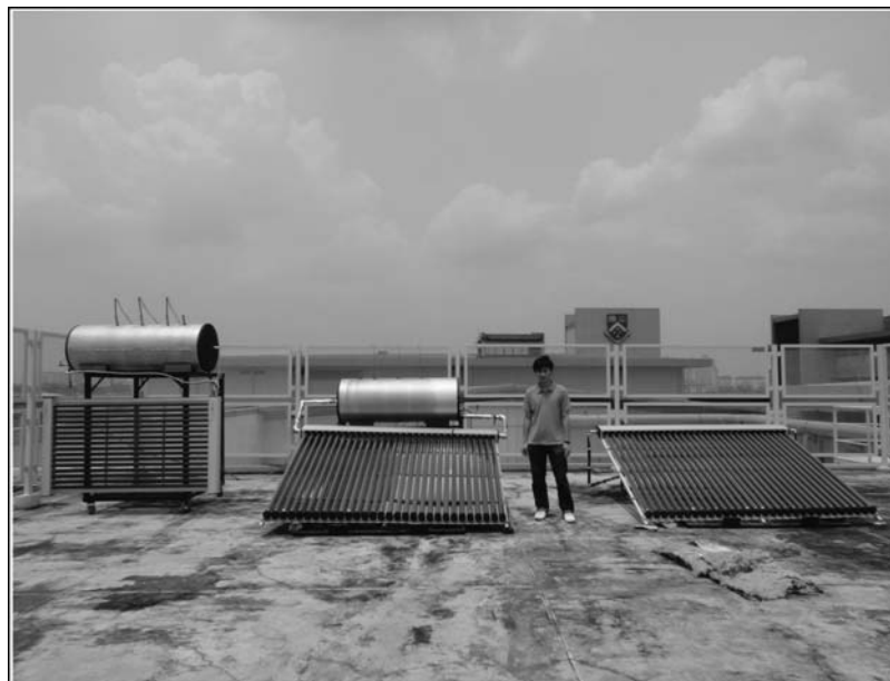
Figure 3. U-tube and heat pipe solar water heaters set-up.
