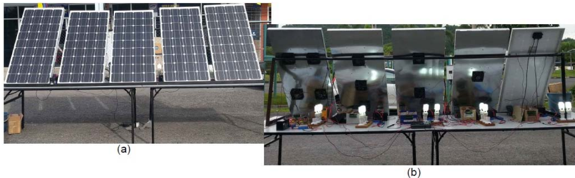
Figure 3. The outdoor experimental of PV system with and without cooling system
