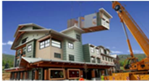
Figure-1. The modular building has the same features as a conventional building [10].
