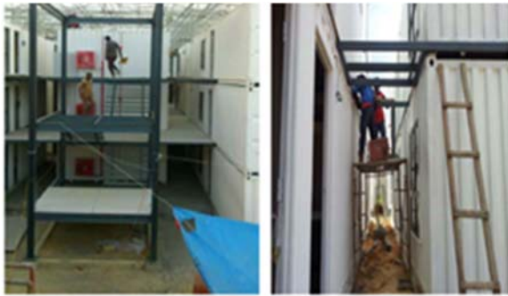
Figure-20. Site installation of staircases, floor joists and other structures between stack shipping containers.
