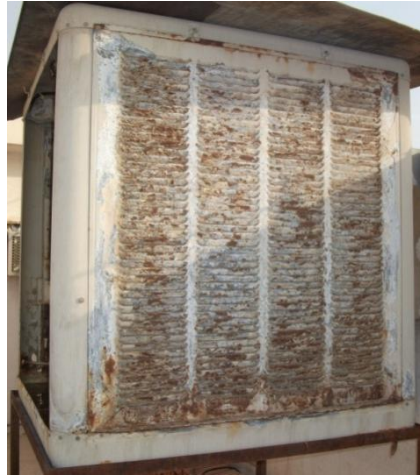
Figure (2): The affect of the cumulated salt on the evaporative cooler (outside the cooler)
