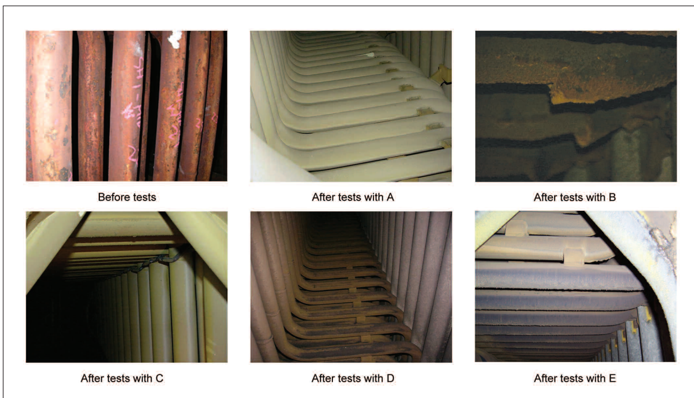
Figure 4: Superheater tubes before and after the tests.
