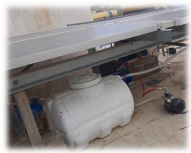
Fig. 13. Water tank used in the project.
