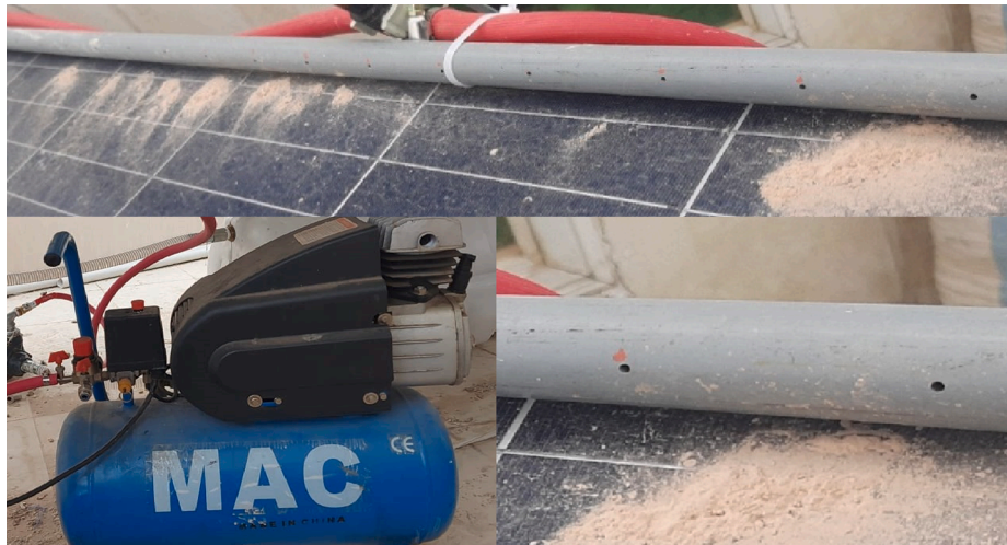
Fig. 11. Air cleaning components utilized in intelligent cleaning system pilot project.
