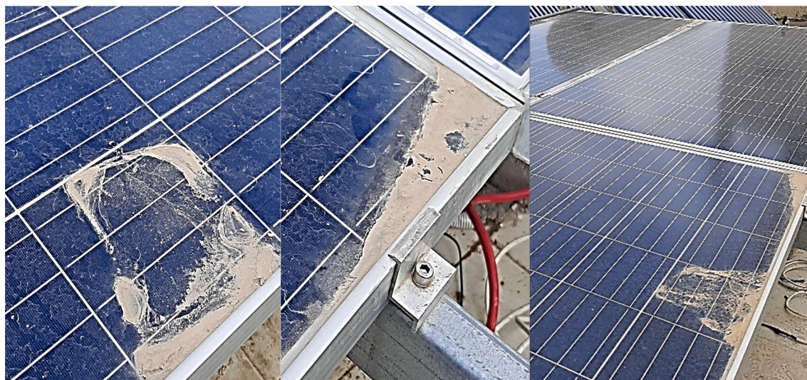
Fig. 2. Exemplary photographs of soiling mineral dust in Al-NAJASHI mosque, Al-Salt, Jordan.
