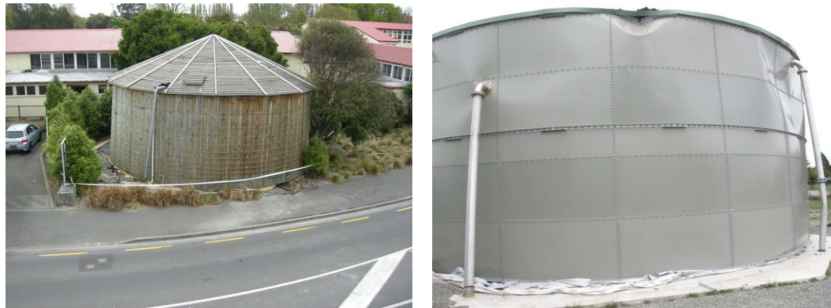
Fig. 1 Foundation sliding (right) and wall damaged due to sloshing motion (left) in Darfield earthquake (2010) (Courtesy of Timbertanks)
