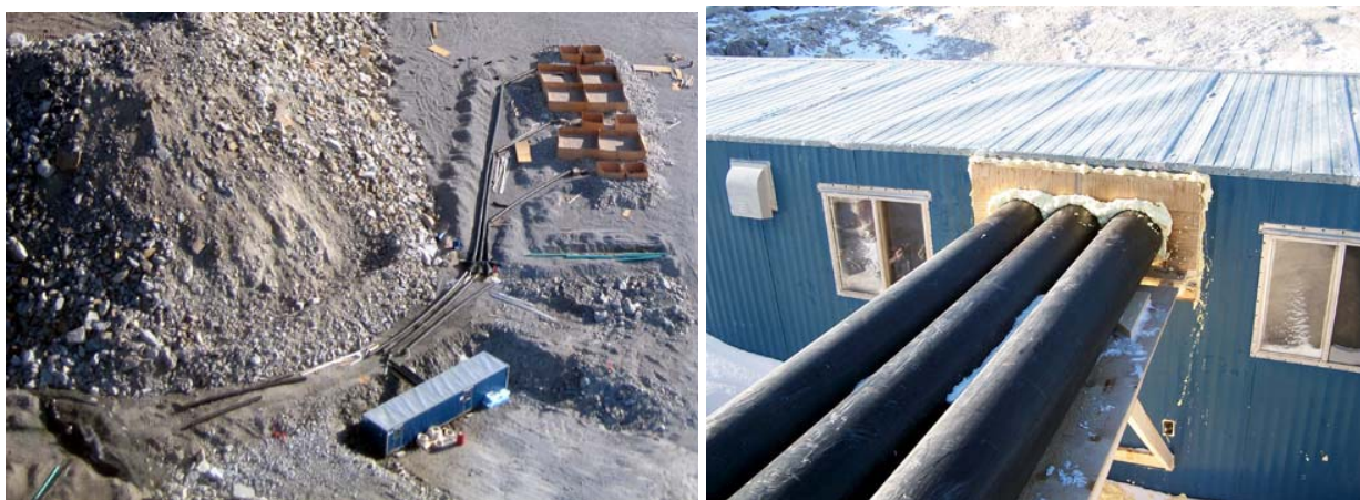
Figure 9. Photo to the left shows cluster lysimeter drainage pipes directed into the instrumentation shack. The instrumentation shack is situated between the Type I and Type III rock pads. The photo to the right shows lysimeter drainage pipes entering the instrumentation shack.
