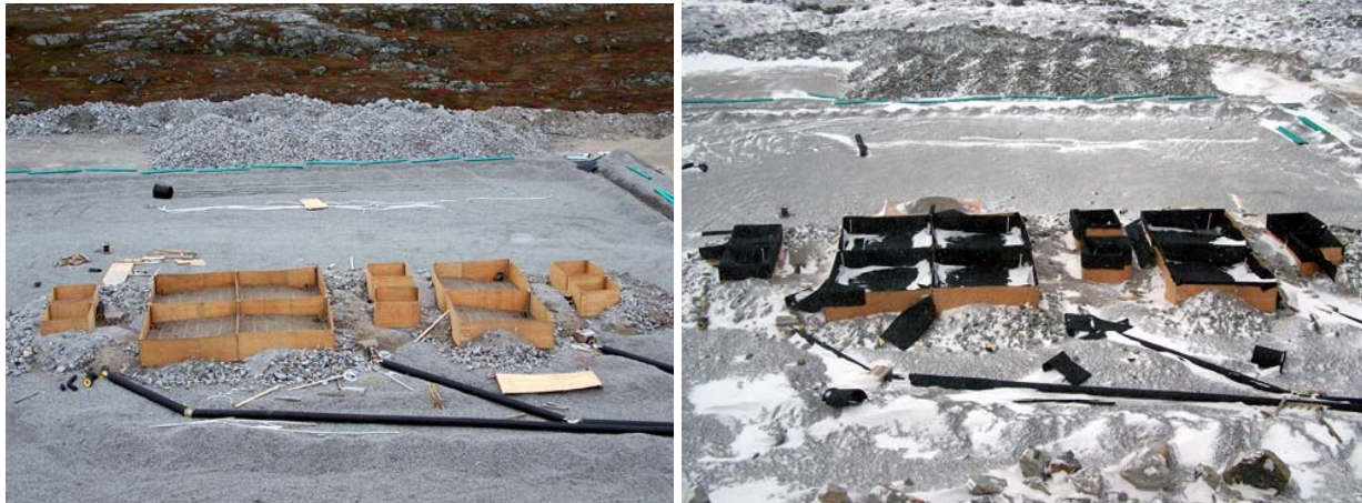
Figure 8. Photo to the left show three lysimeter clusters constructed over the Type III test pad. Loops of wire on the lysimeter pads are heat trace cable. The black 10-inch insulated pipe house the 1.5-inch drainage pipes exiting from each lysimeter. The photo to the right shows a completed cluster lysimeters with an impermeable HDPE liner.
