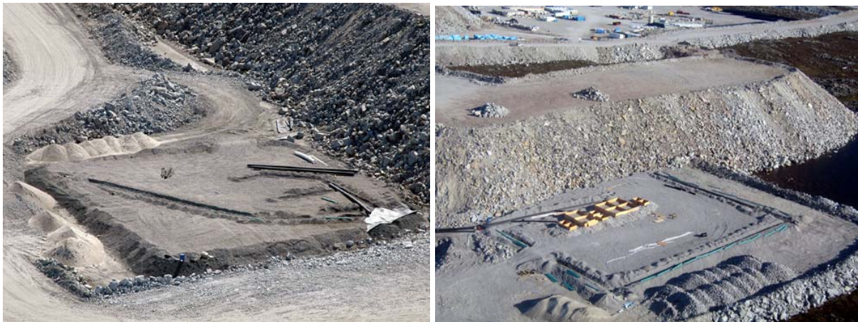
Figure 7. Photo to the left shows the basal drainage ditch excavated diagonally across the center of the Type I pad exiting through the SW corner. Photo to the right shows the basal drainage ditches excavated around the perimeter of the Type III pad exiting through the NE and NW corners.
