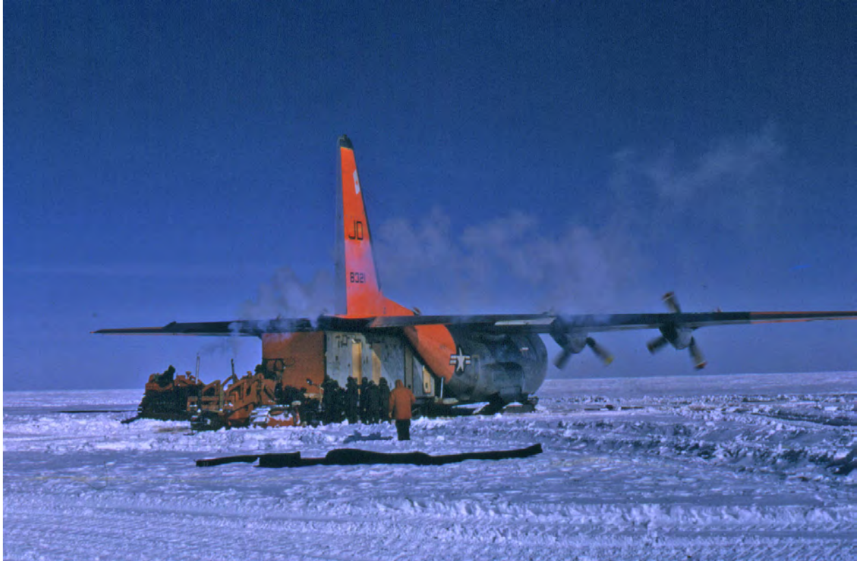
Off loading the first section of the main camp building at Plateau Station January 1966
