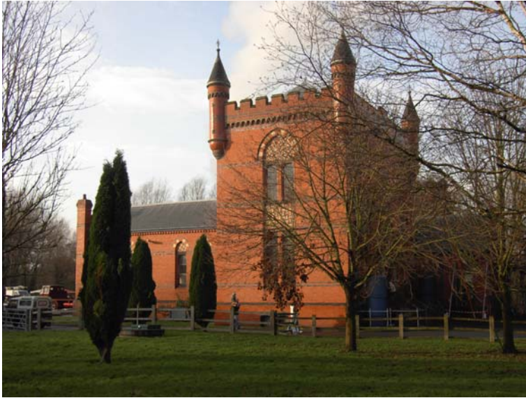
Fig. 1. The Bratch groundwater pumping station, built in Victorian gothic style by the Bilston Corporation, 1895 (courtesy of Friends of The Bratch).
