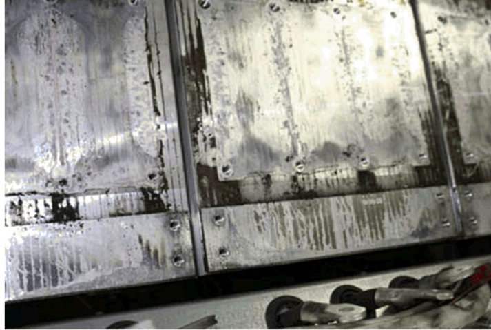
Figure 8: Heat sink of a failed inverter with no thermal grease remaining below the power module's hot spot
