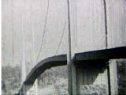
Figure 1: the Tacoma Narrows bridge hitting resonance, from Physics: The Core (Saunders) {2} much more exciting — and understandable if the sound of wind is included.
