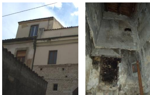
Figure 9: Weaknesses in block 69: standing out body and lack of floor.
