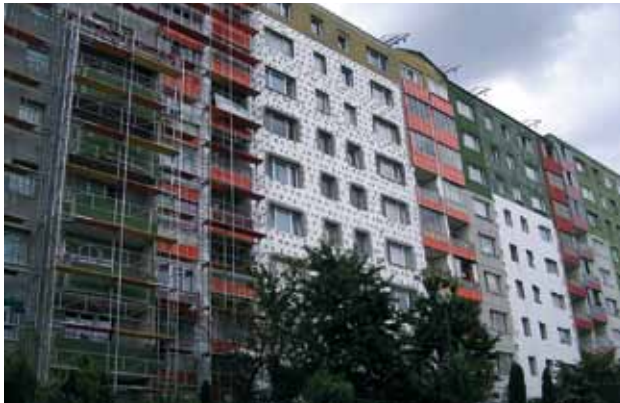
Fig. 1. A lot of bat roosts in buildings is destroyed by insulation works (photo Roman Lehotský).
