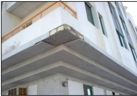
Figure 9 Falling of External Marble Cladding
