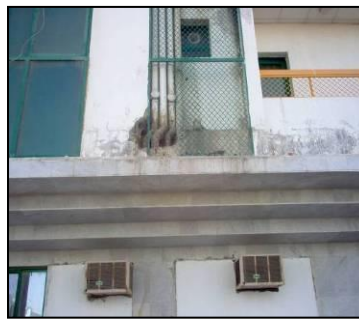
Figure 10 Concealed Sanitary Pipes
