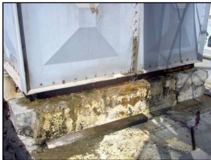
Figure 7 Damaged Water Tanks
