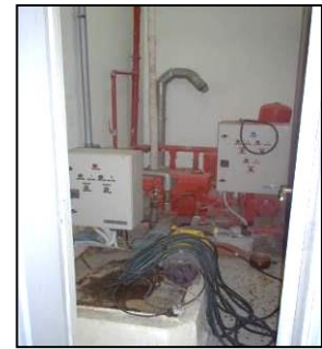
Figure 11 Congested Pump Room
