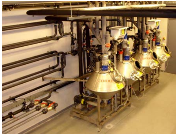
Figure 1 : The liquid feeding system used (ACEMO, France). Fermentation tanks have a working volume of 70 liters and pipelines are 25 meters long.
