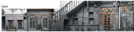
Court New Partition Wall Non Load Bearing Arches Electricity panels Additional elements and Doors to close the arches
