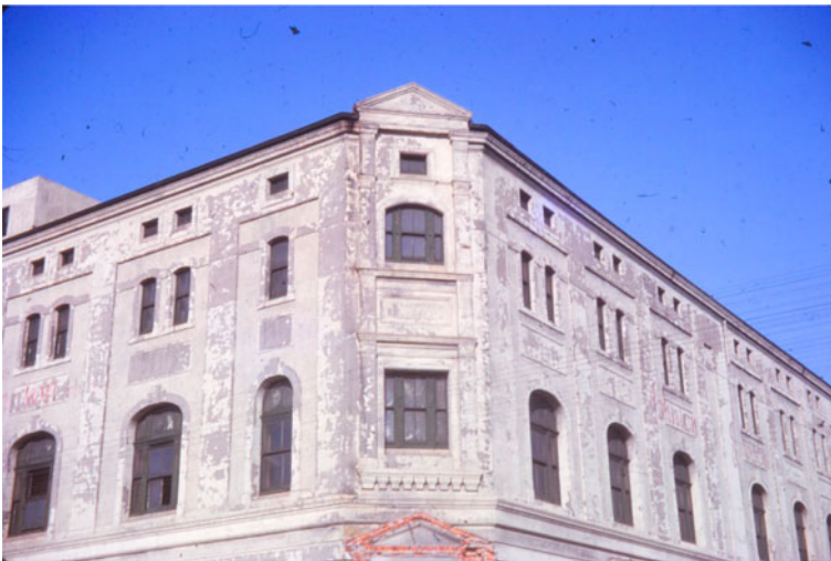
Figure 9. The Johnson & Johnson building in decay.
