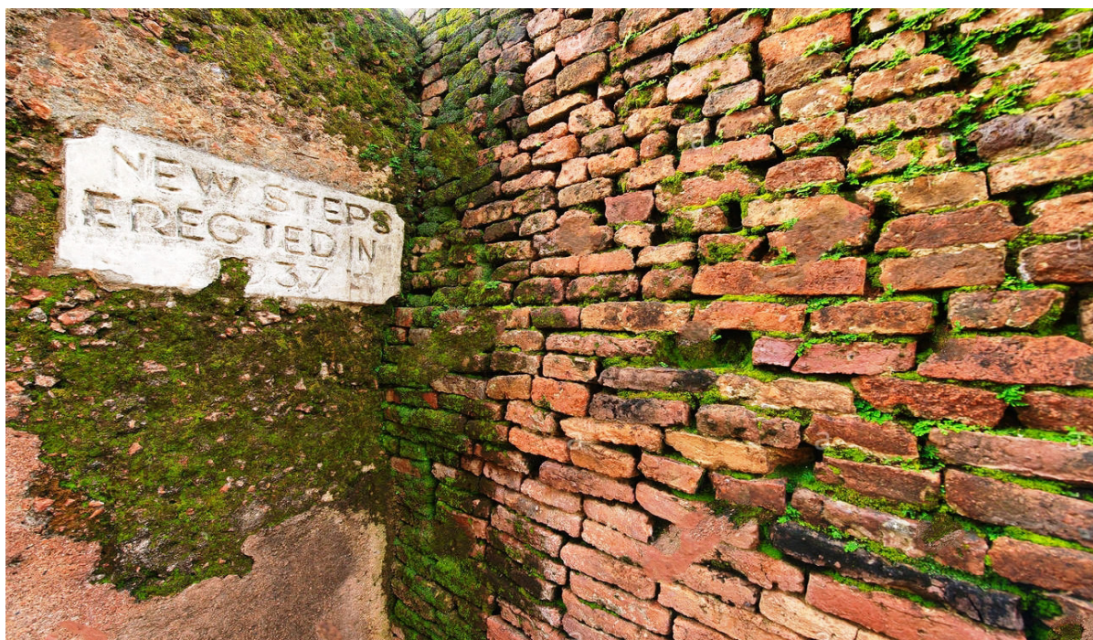
Figure-8: Damage caused by 1934 Earthquake to Maniyar Math.
