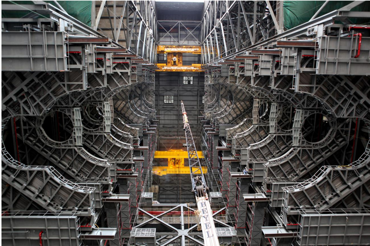
Figure 2. New work platforms have been installed in Kennedy Space Center's Vehicle Assembly Building for stacking the SLS vehicles
