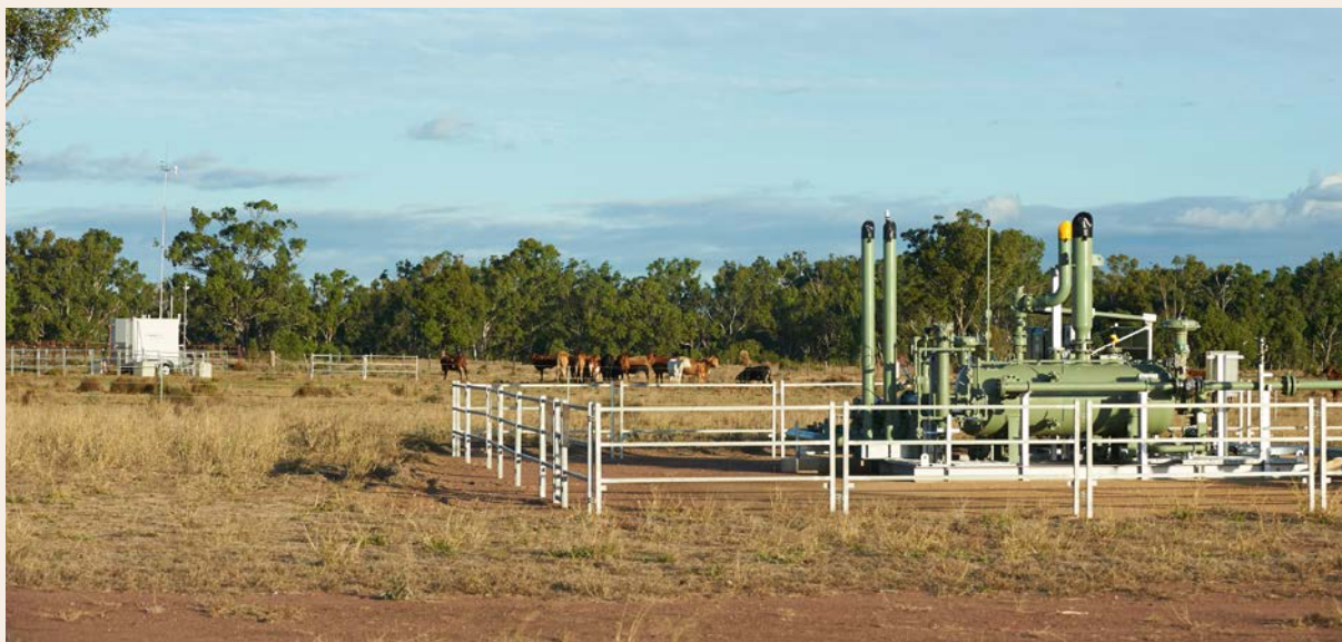
Wells and air quality station at Hopeland, Queensland
