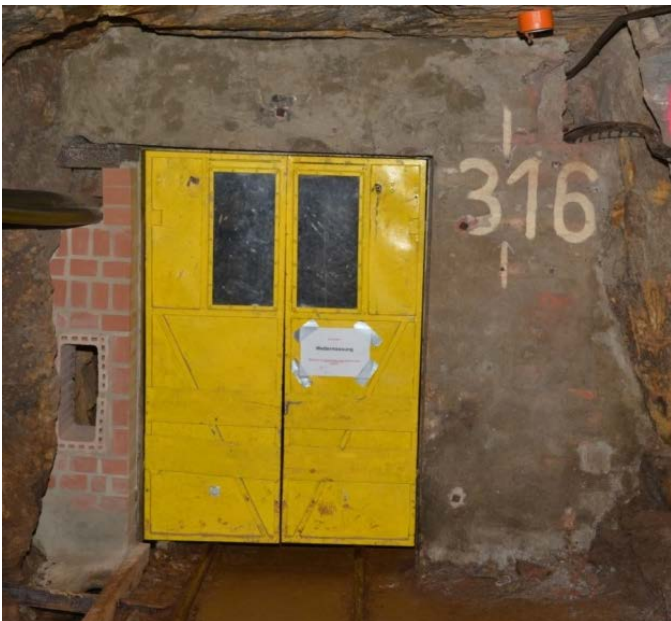
Figure 2. Concrete and brick stopping with steel door and a fixed regulator on the left side.
