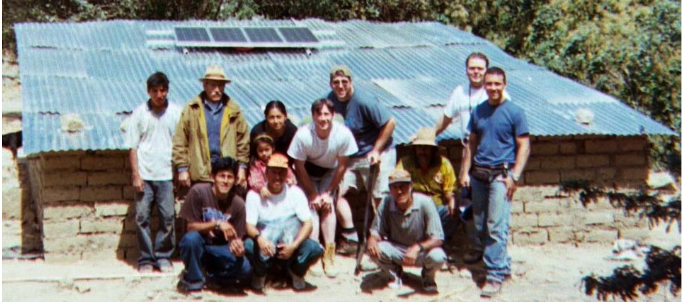
Fig. 6 Adobe shelter with PV modules mounted showing some of the authors and villagers.
