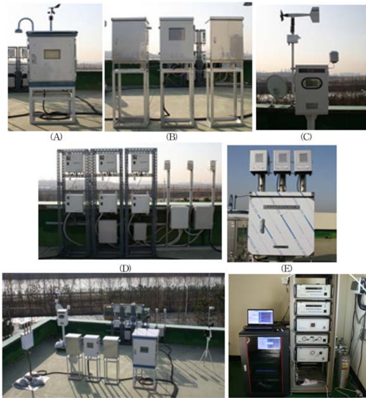
Fig. 2. Odorous gas sensors and NH 3 , H 2 S measuring equipment.
