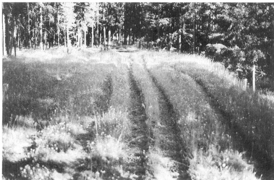
Figure 2. Open trailside vegetation and flat sideslopes invite hikers to wander off the trail tread, resulting in trail widening and multiple treads
