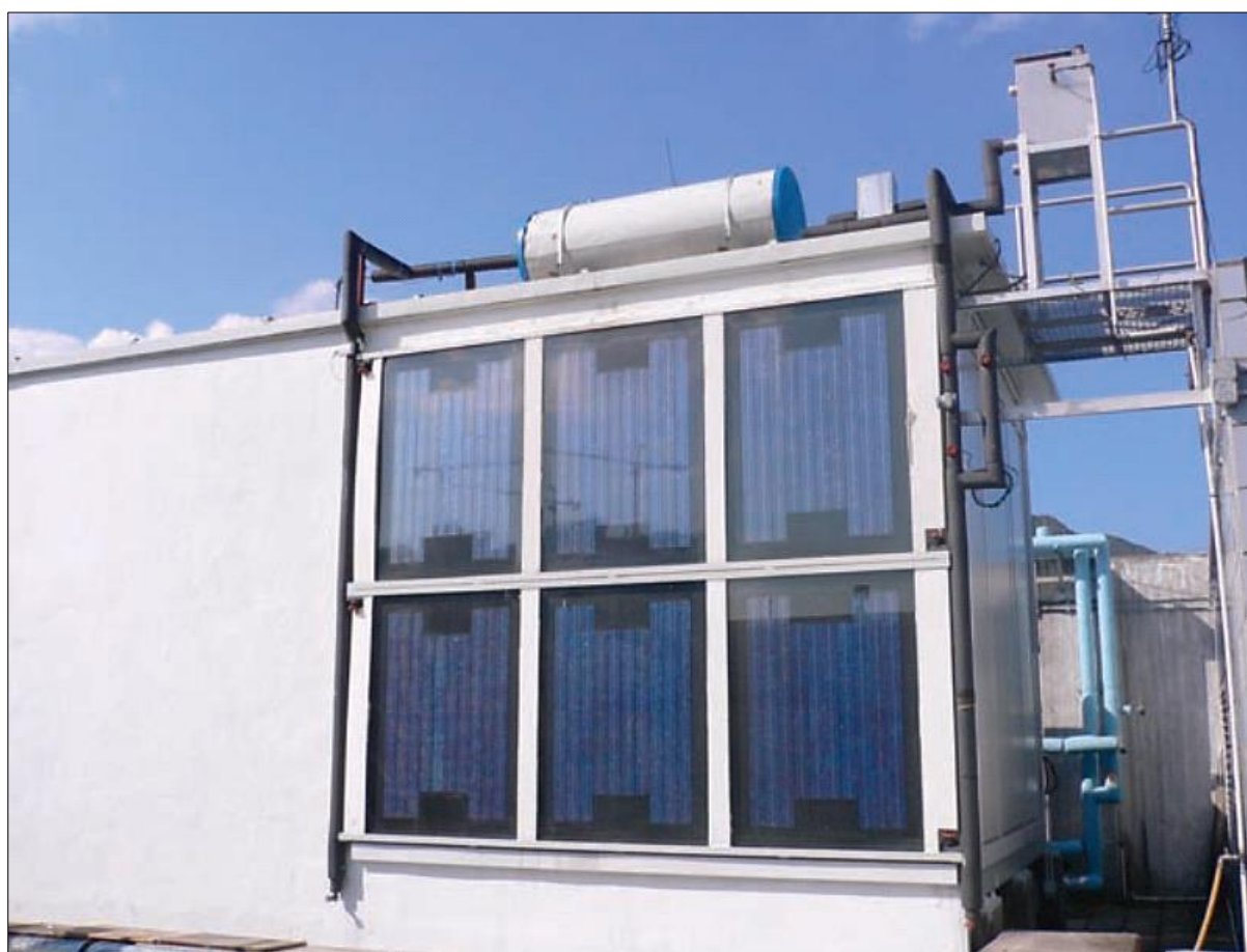
Fig. 24: Experimental Setup of Building Integrated Photovoltaic/Water Heating System at City University of Hong Kong [12].
